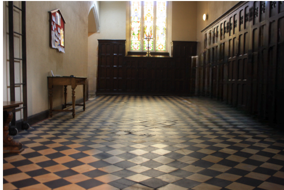
Cloister Corridor with uneven tiles on-route to the Chapels
